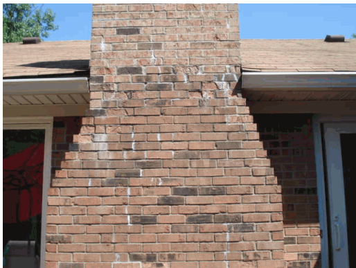
BRICK SCALEING ON REAR CHIMNEY
