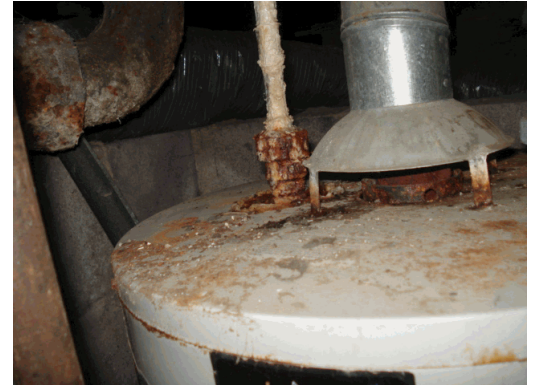
RUSTED LEAKING WATER PIPE AT WATER HEATER
