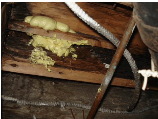
EVIDENCE OF MOISTURE &amp; ROT IN SUB
