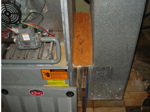
RUST ON DUCT WORK CAUSED BY LEAKING AC COIL.
