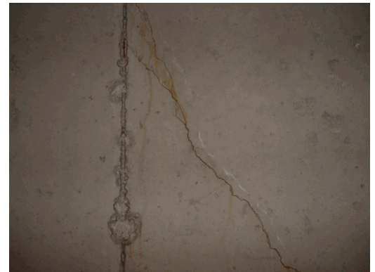
EVIDENCE OF WATER INTRUSION IN BASEMENT WALL
