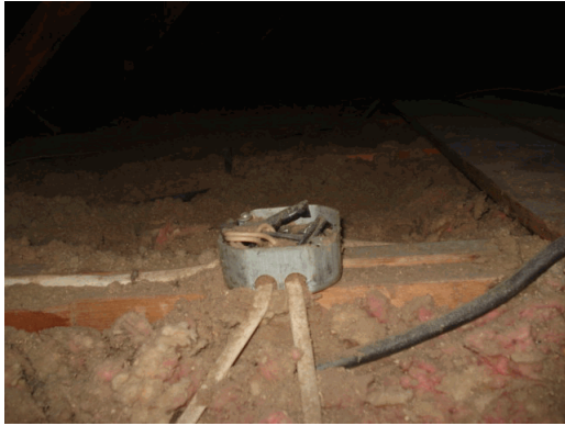
ELECTRIC JUNCTION BOX WITH NO COVER
