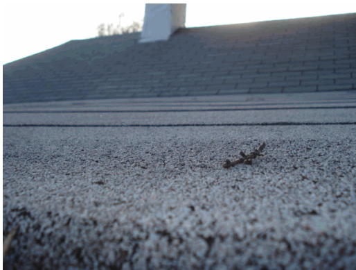
EVIDENCE OF ROLL ROOFING BEYOND DESIGN LIFE
