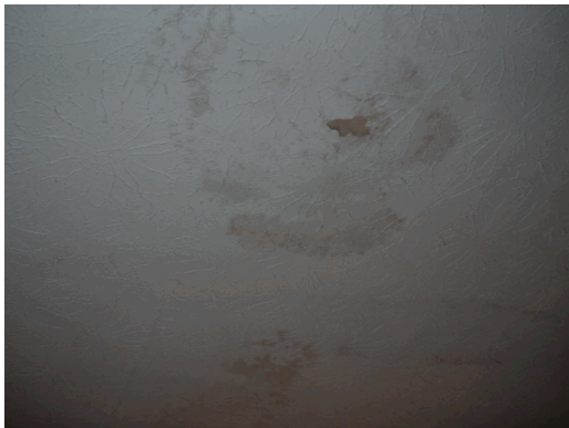
EVIDENCE OF WATER INTRUSION IN CEILINGS
