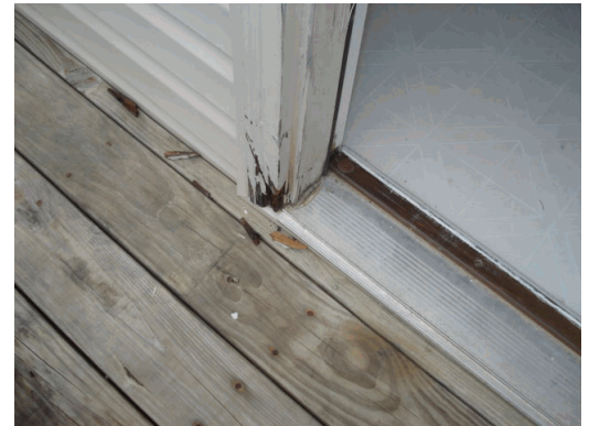
MOISTURE DAMAGE TO WOOD TRIM AT DECK DOOR
